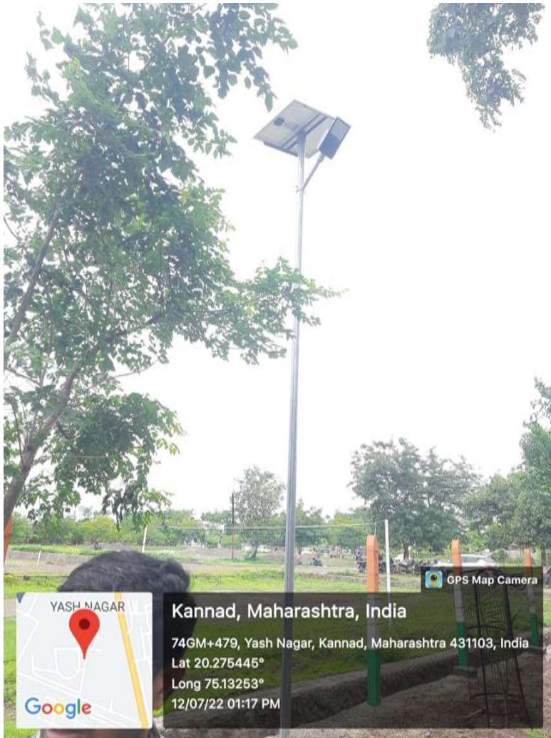
5. Solar Energy LED Street Light
