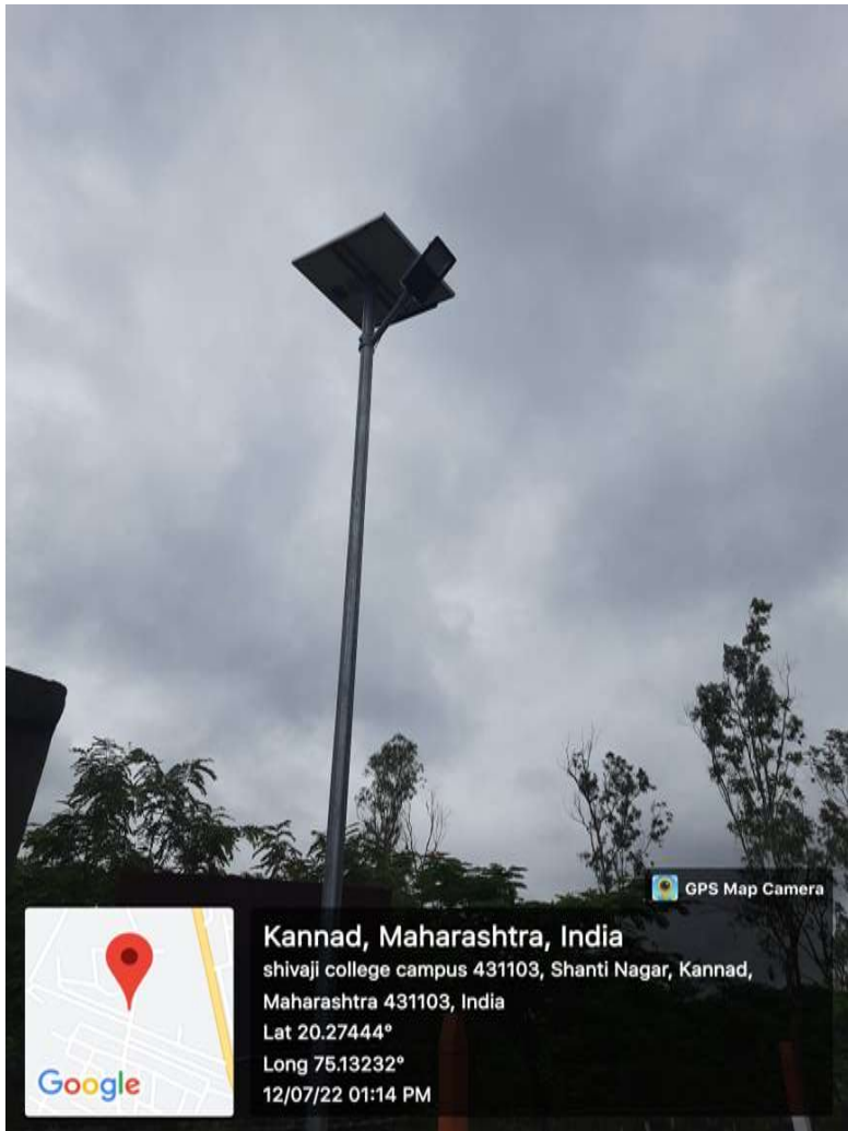
3.Solar Energy LED Street Light
