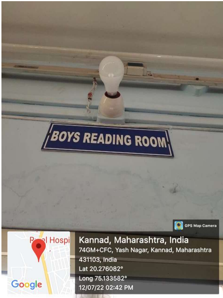
19. LED Bulbs in Reading Room
