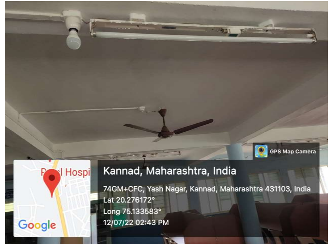
20. LED Bulbs in Reading Room
