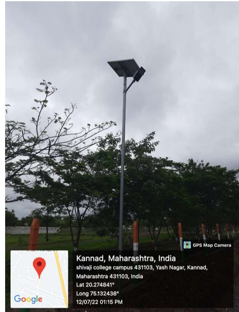
4.Solar Energy LED Street Light
