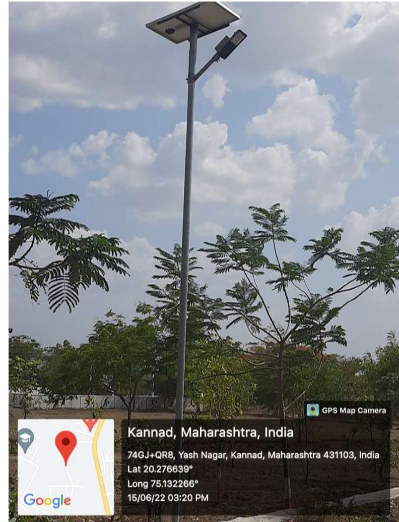
2.Solar Energy LED Street Light
