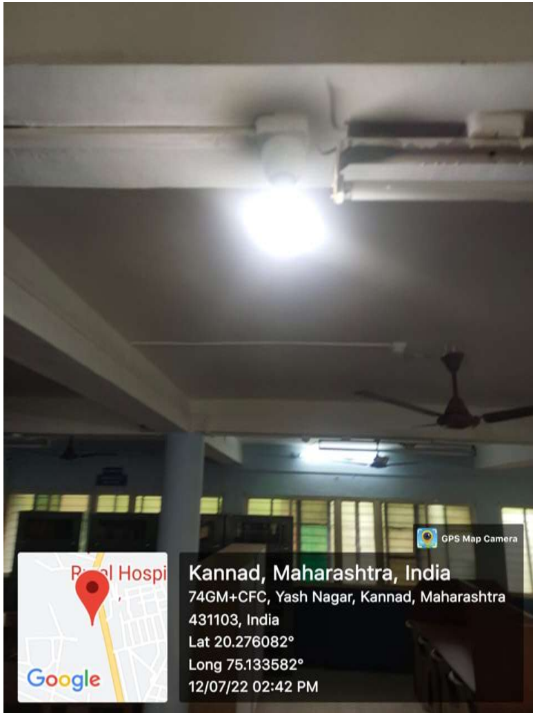
21. LED Bulbs in Reading Room
